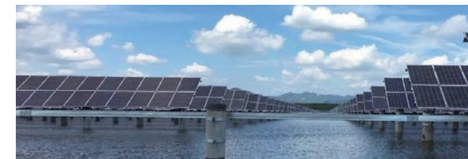
Pile-based fixed photovoltaic power station
